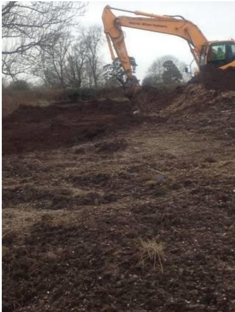
Figure 13: Capping the excavated material with 20cm of material to fulfil the local enforcement notice and planning condition
