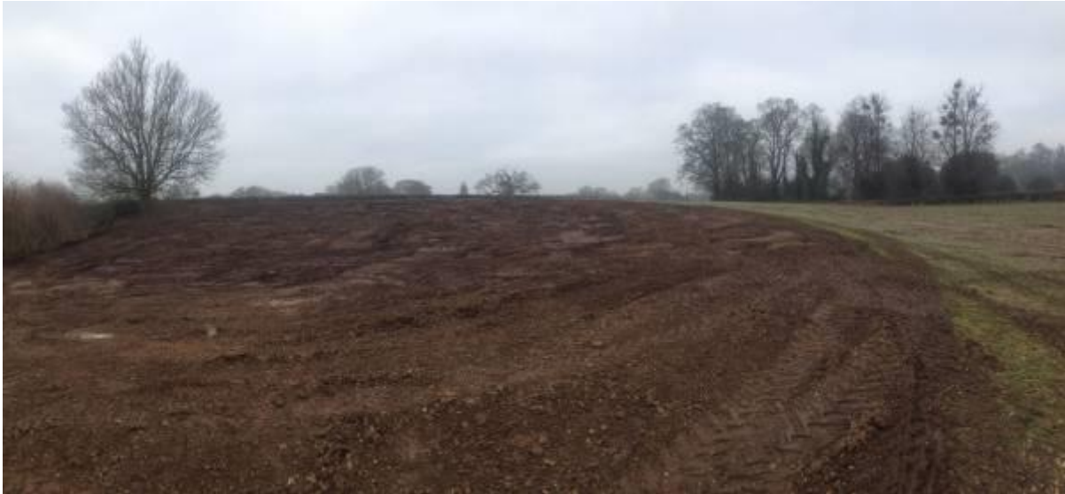
Figure 14: The hollow after capping work ready to be seeded in the spring.
